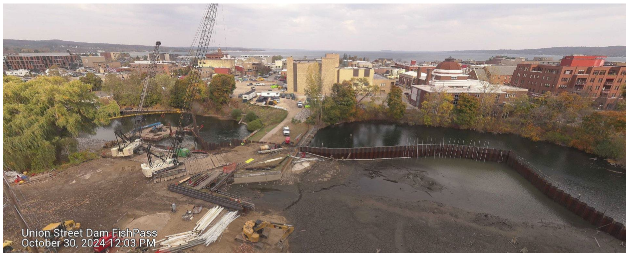
Figure 1. Image from the FishPass time-lapse camera: October 30, 2024 – 3:00 PM showing the sheet pile cofferdam upstream of the dam (right side of image) and continued installation of the downstream portion (left side of image).
